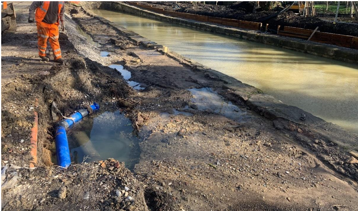
Figure 1: Results of the explosion with several square metres of soil blown out exposing the pipes.
